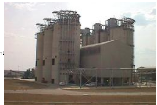
Ash storage silo with pneumatic conveying piping and dust suppression filters
