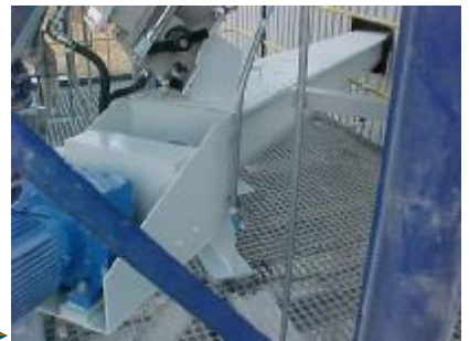
Screw Conveyor transporting material from a Silo to a Bag Filling Plant
