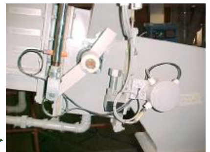
Flow Control Valve with Proximity Switch and adjustable mechanical stop. Note the aeration point
