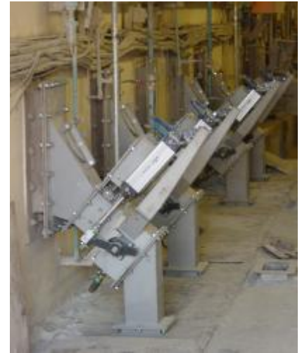
Silo Discharge arrangement with Flow Control Valve & Knife Gate Valve
